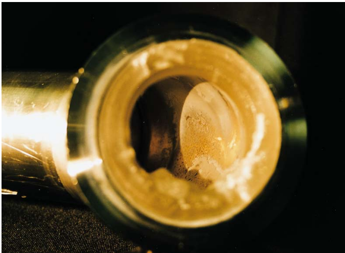
Fig. 1: Illustrates the reduction in tube cross section due to aluminum chloride build up in an insufficiently heated tube.
